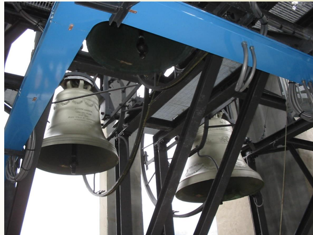
CAVI in cella campanaria
